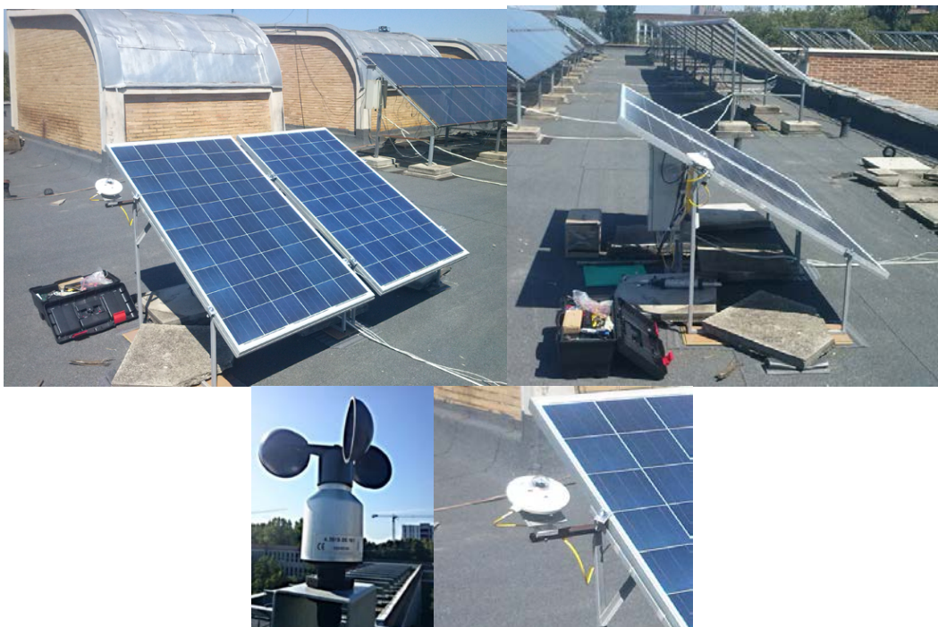
Images with the experimental system installed on the roof of the Faculty of Electrical Engineering
