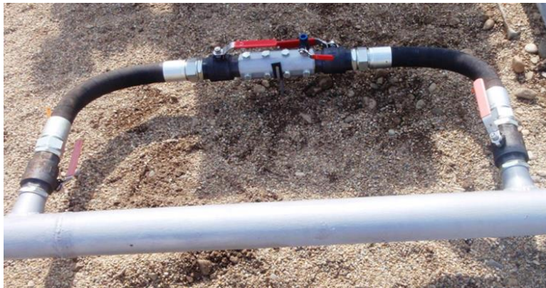
Fig.3 The device installed in location no.1
